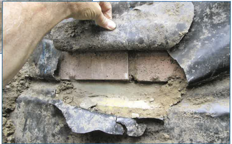
Figure 8 – Damaged caulking at transition between the reddish precast panels (atop steel framing) and underlying cast-in-place concrete wall. A probe inserted into this hole readily extended into the boiler room at the area of water staining seen in Figure 4.
