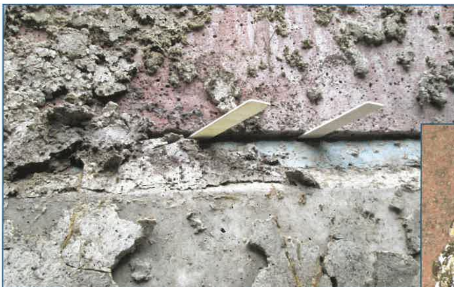
Figure 10 – The caulk joint between the two wall systems was not watertight due to failed bonding at the precast panels.
