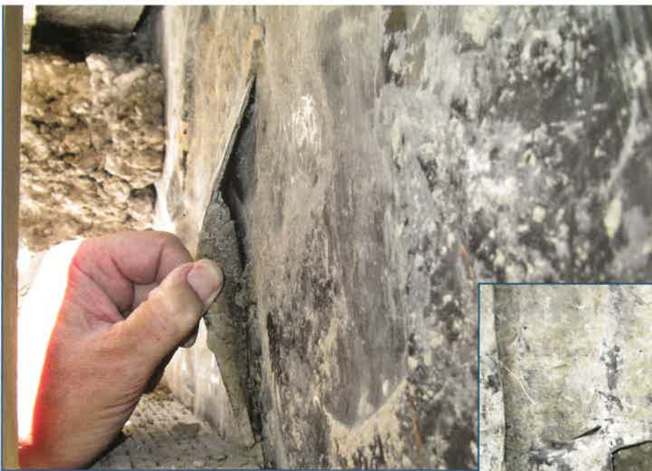
Figure 11 – Multiple breaches in the membrane due to damage during backfilling were observed at all levels of the excavation.
