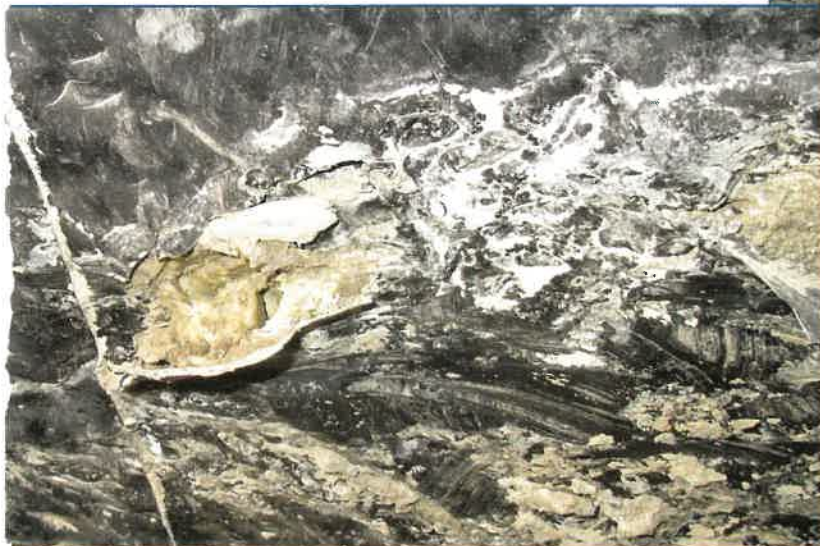
Figure 13 – (below) Near the bottom of the excavated trench, breaches in the waterproofing still remained prevalent.
