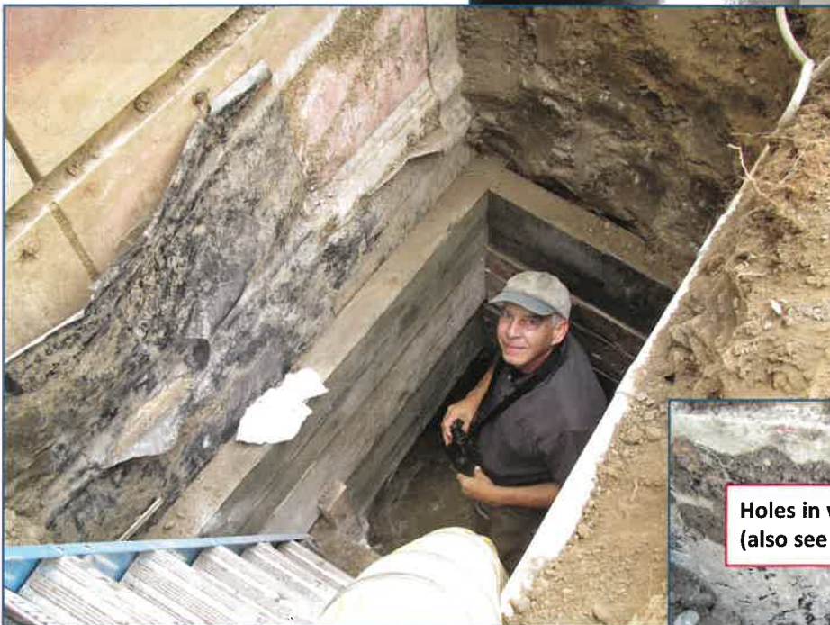
Figure 5 – Upon commencing the excavation process, a raggedy, poorly attached, and extensively torn sheet waterproofing membrane was exposed. (The missing section at the top of this photo was extracted by our crew for sampling purposes.)
