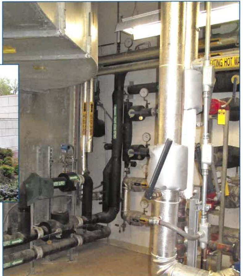
Figure 2 – A cast-in-place concrete wall encloses a 70-ft.-long boiler room that serves the entire campus.
