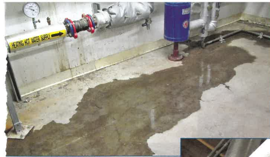
Figure 3 – Even during dry weather, groundwater infiltrated the boiler room at floor-to-wall transitions. The water stains at the lower cast-in-place wall (at left) resulted from leakage occurring at the top of the concrete wall (see Figure 4).
