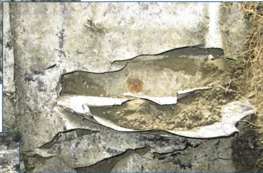
Figure 12 – Contractor(s) severely damaged the sheet membrane during the backfilling process.
