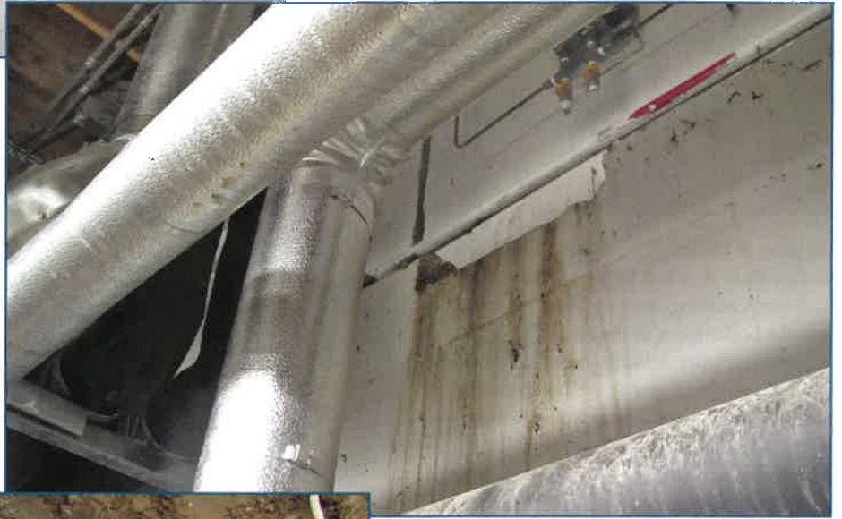
Figure 4 – During rain events, water flooded down from the top of the cast-in-place concrete wall, which commences 20 in. below grade. (The precast panels above are attached to the cast-in-place concrete walls with steel brackets.)
