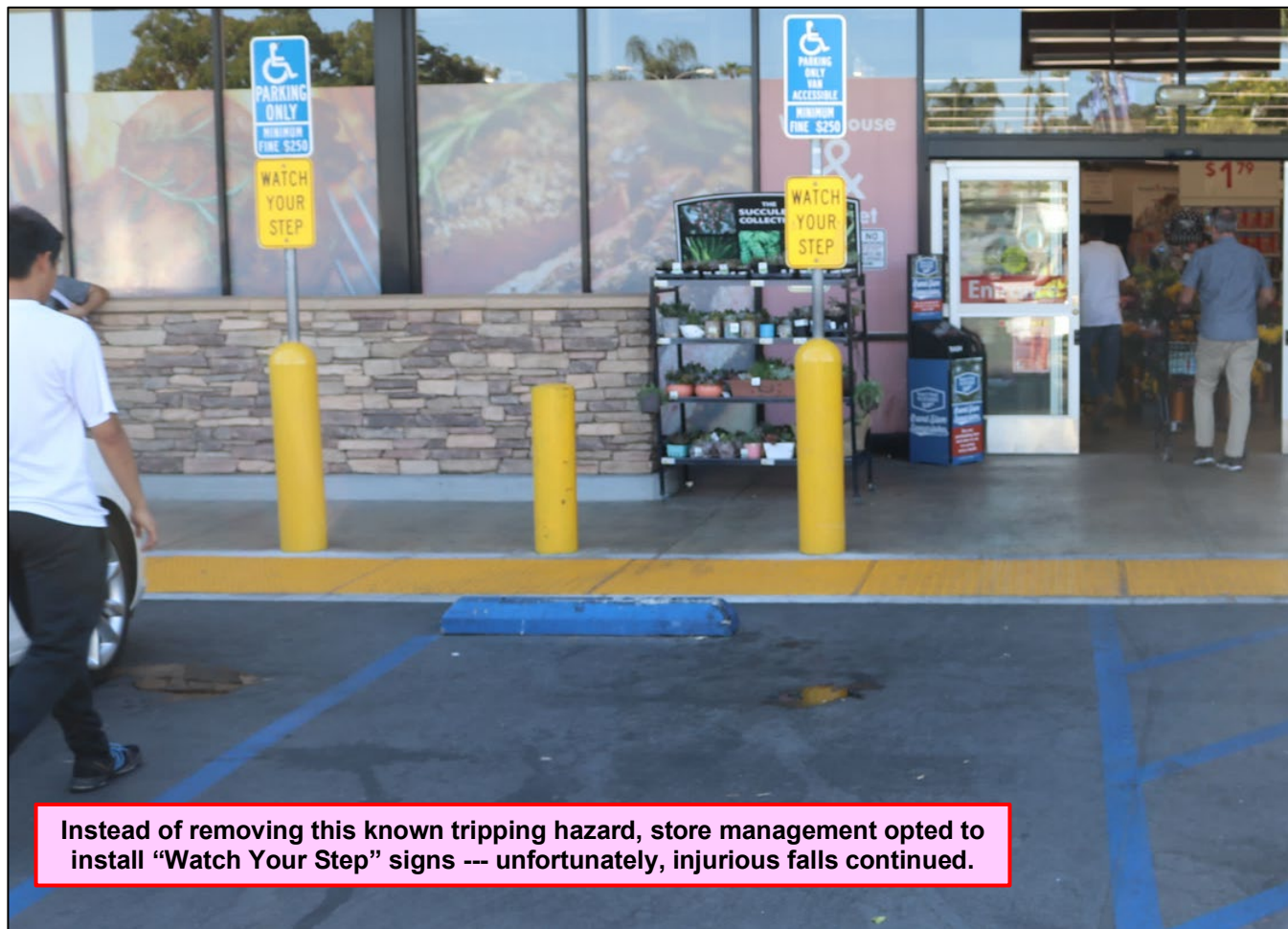
Photo 2 – At this grocery store in Southern California, a primary route of pedestrian travel from the parking lot toward the entry doors led across this wheel stop --- what could go wrong?
